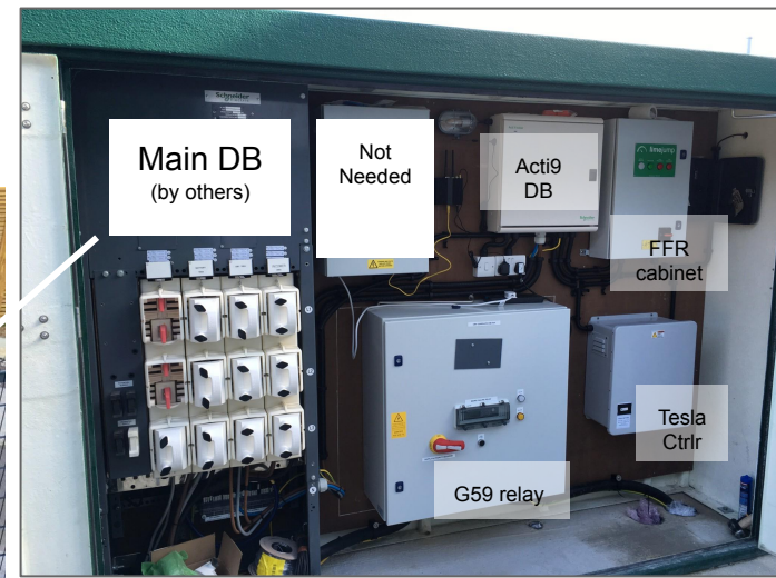
Figure. Battery Controls Equipment
